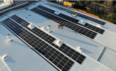
Bulgaria Industrial&Commercial Energy Storage System
